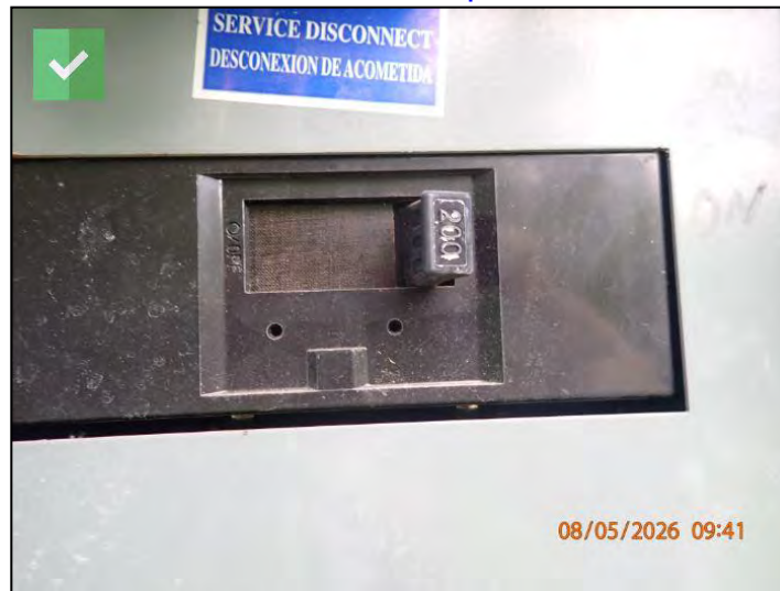
200 Amp (Main Panel)
