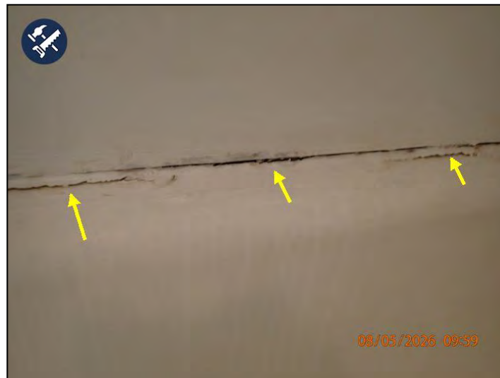
Failing Sealant/Caulk (Multiple Locations)
