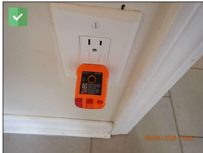
GFCI Reset Location: Within Receptacle
