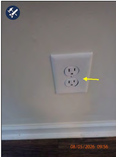
Loose/Improperly Installed Outlet(s) (Living Room)
