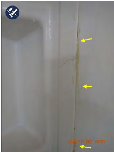
Failing Sealant/Caulk (Guest Bathroom)
