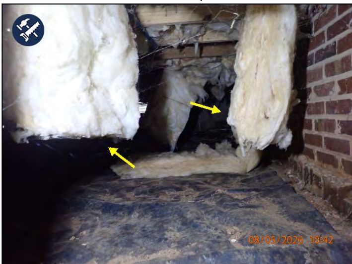
Failing Insulation (Multiple Locations)
