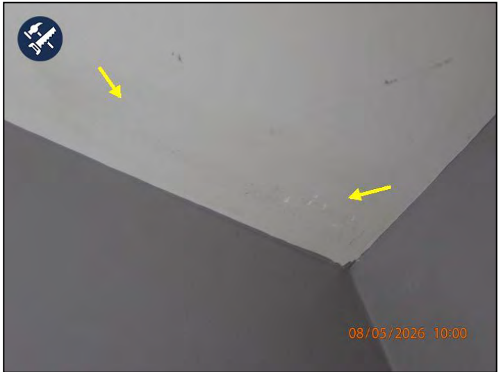
Past Repairs (Unable To Determine If Professional) (Multiple Locations)
