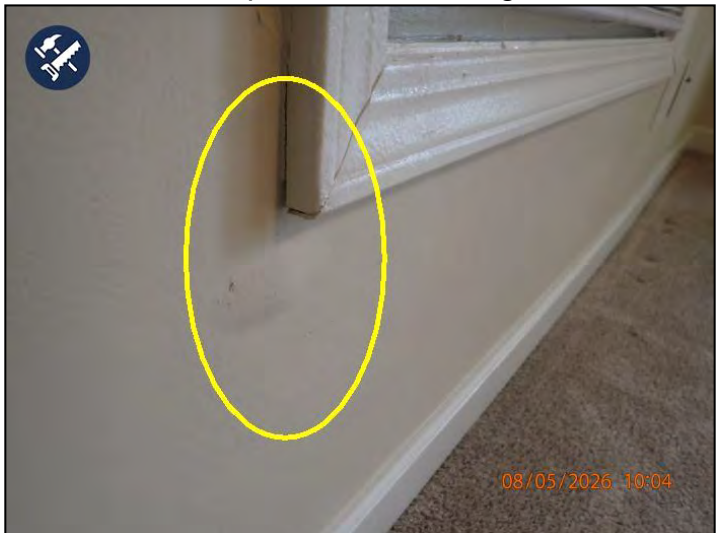
Past/Present Moisture Intrusion (Multiple Locations)
