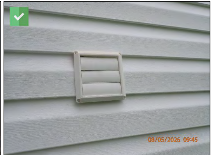
Vents To Exterior
