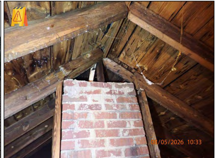
Abandoned Chimney (Unable To Determine If Properly Capped/Sealed Due To Height Restrictions)
