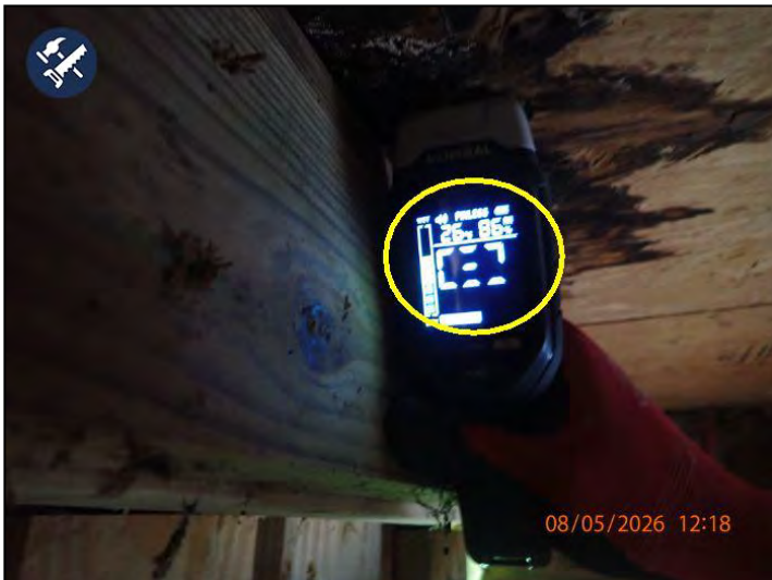
Moisture Intrusion/Damage (Beneath Water Heater)
