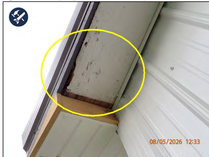
Damage/Deterioration (Multiple Locations)
