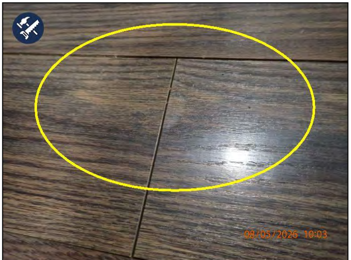
Not Level/Buckling Flooring (Multiple Locations)
