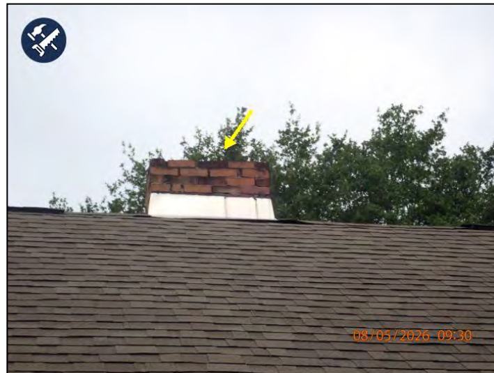
Missing Spark Arrestor/Rain Cap
