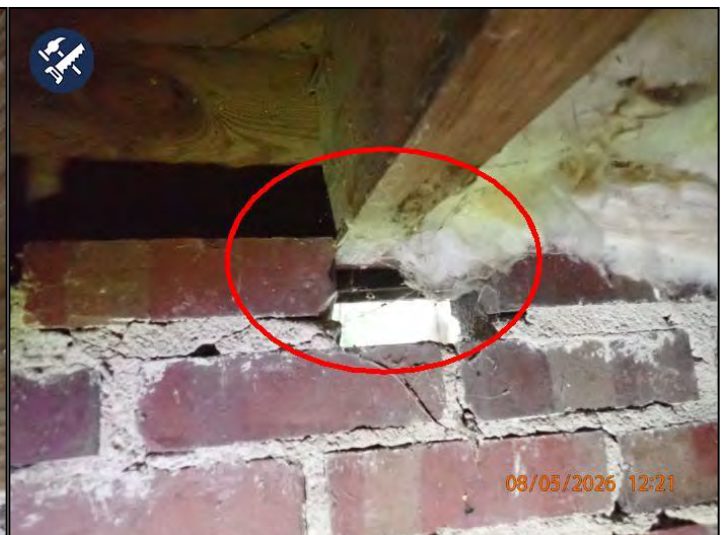
Floor Joist Not Supported (Rear Right Of Structure)
