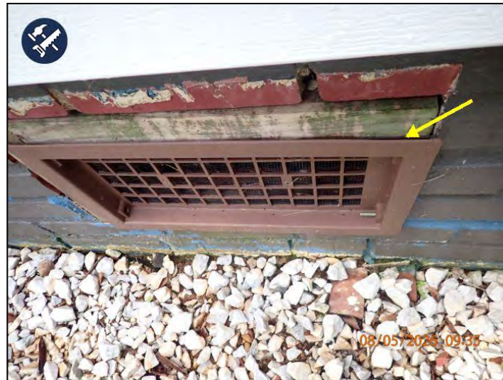
Not Secure To Structure (Multiple Locations)
