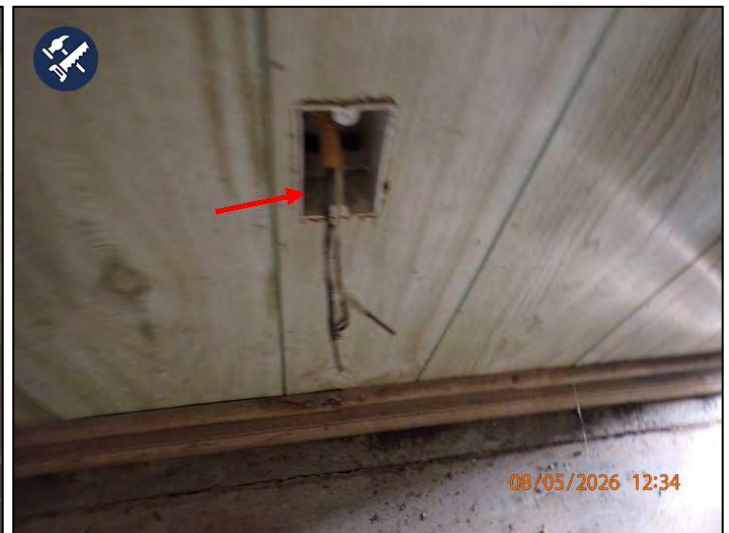
Open Junction Boxes (Multiple Locations)
