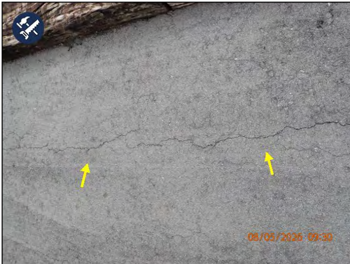
Typical Cracking (Walkway) (Multiple Locations)
