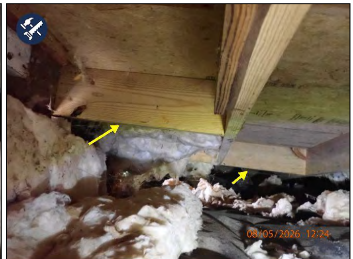
Past Repairs (Unable To Determine If Professional)
