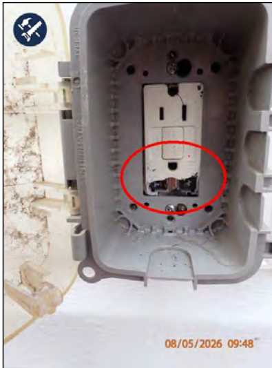
Damaged Receptacle (Left Of Structure)
