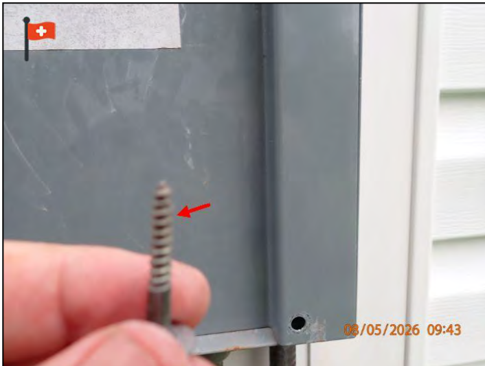
Wrong Fastener(s) (Main Panel)
