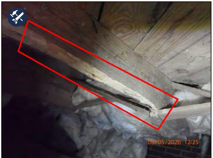
Deterioration To Sub Floor (Multiple Locations)
