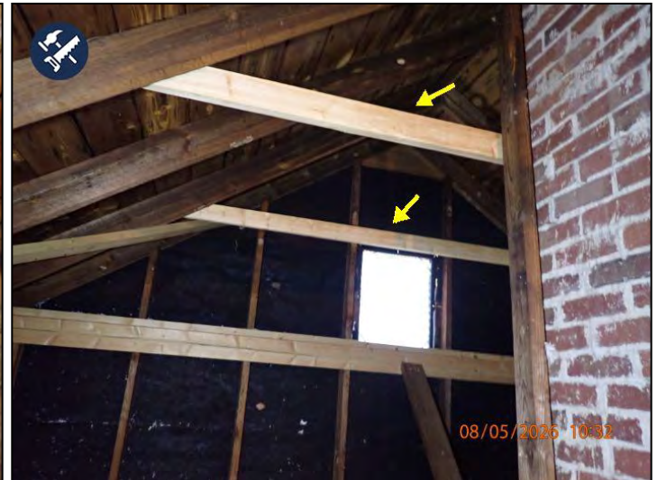
Past Repairs (Unable To Determine If Professional)
