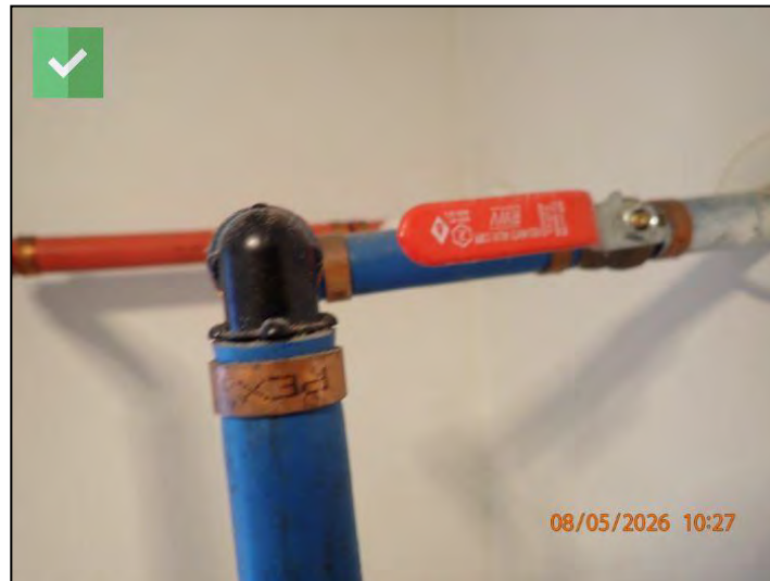
Cold Water Shut Off Valve Present
