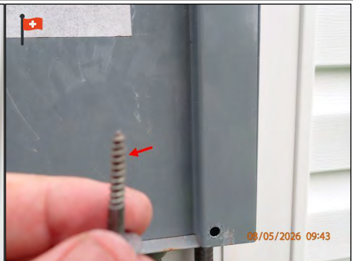
Wrong Fastener(s) (Main Panel)
