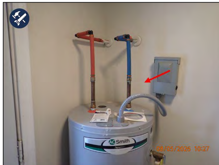
Expansion Tank Missing
