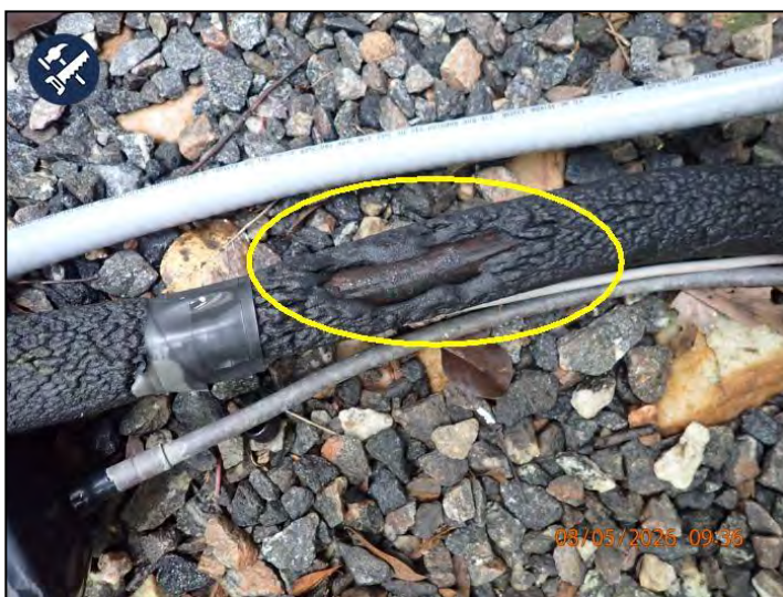
Damaged/Worn (Multiple Locations)
