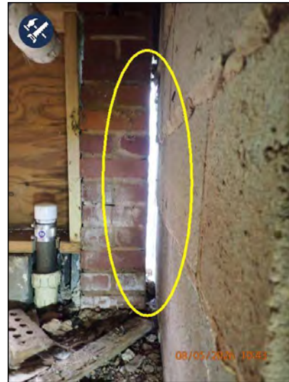
Unsealed Penetration(s) (Multiple Locations)
