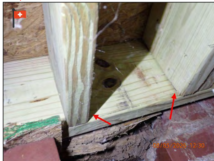
Missing Joist Hangers
