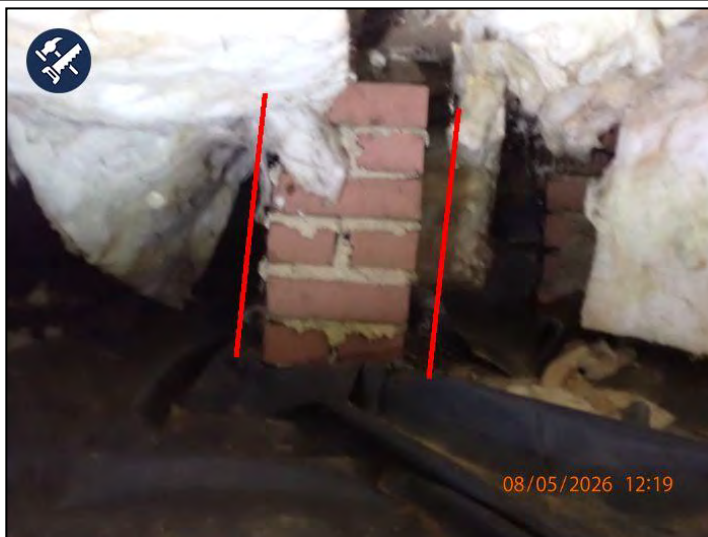
Leaning Pier(s) (Multiple Locations)
