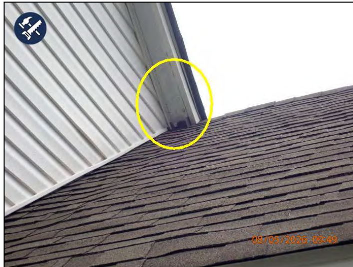
Damage/Deterioration (Multiple Locations)
