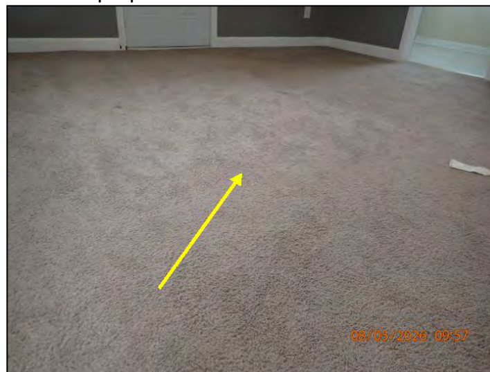
Not Level/Soft Sub Flooring (Multiple Locations) (Primary Bedroom)
