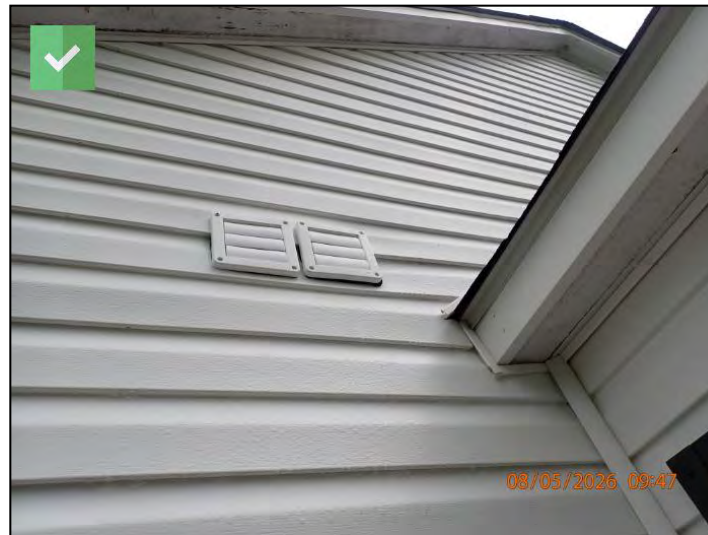
Vented To Exterior
