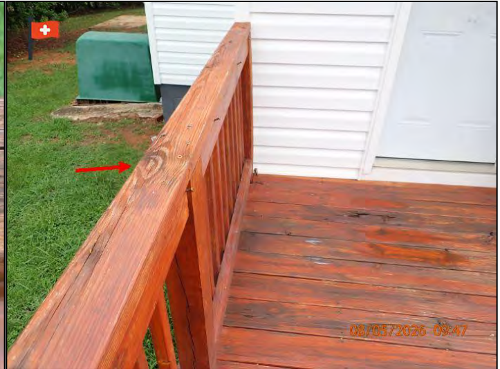
Loose Guardrail(s) (Left Of Structure)
