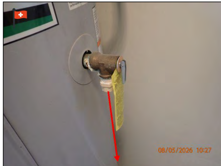
Missing Discharge Pipe
