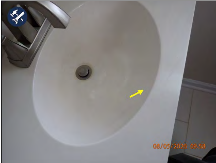
Missing Overflow Drain (Primary Bathroom)
