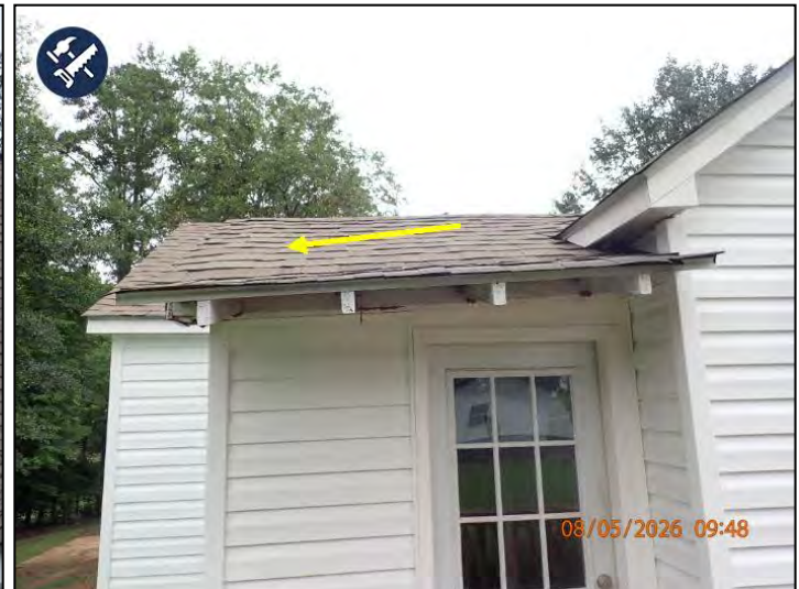
Sagging/Buckling (At Eave)
