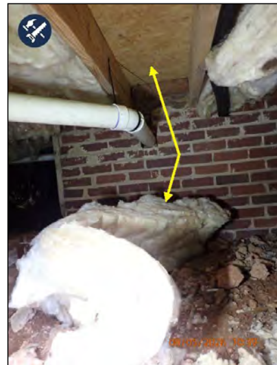
Failing Insulation (Multiple Locations)
