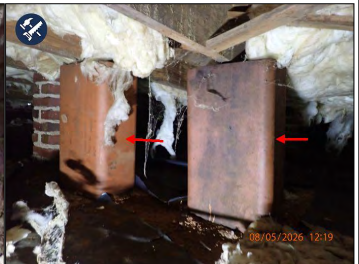
Unprofessional Install (Terracotta Pipes)
