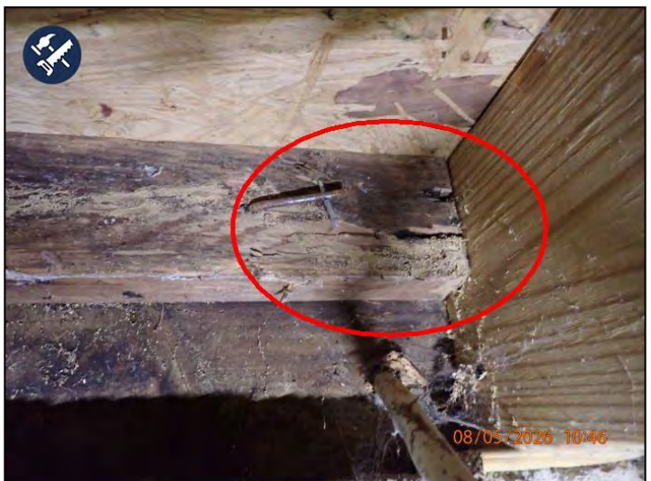
Damage/Deterioration To Band Sill (Beneath Refrigerator, Tested Dry)
