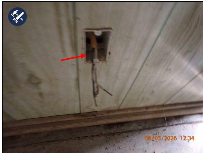
Open Junction Boxes (Multiple Locations)
