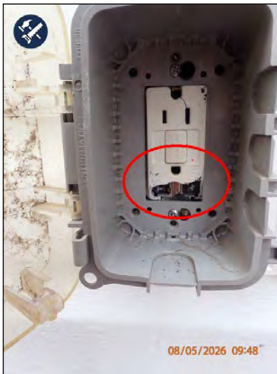
Damaged Receptacle (Left Of Structure)
