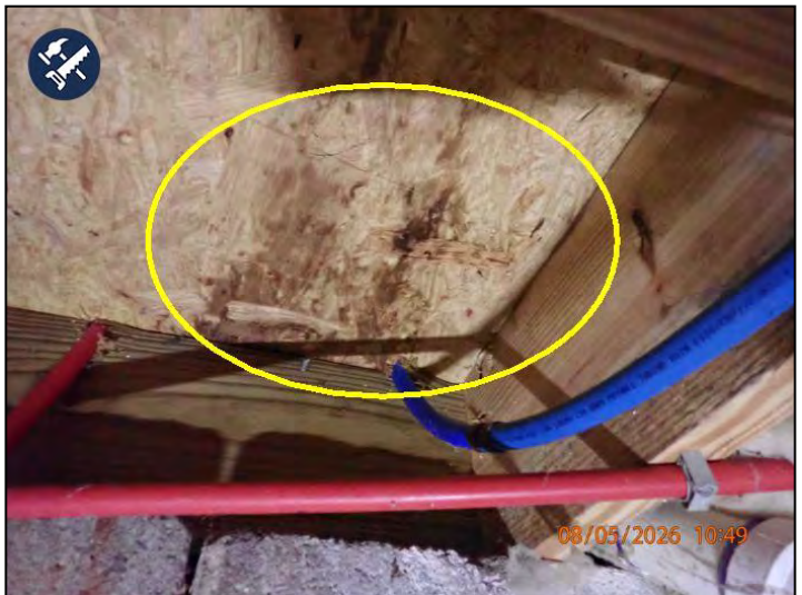
Moisture Intrusion/Damage (Under Kitchen Sink, Tested Dry)
