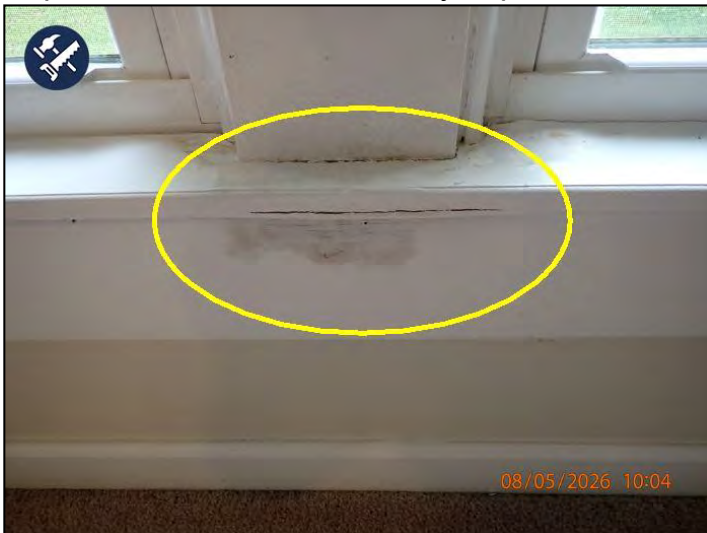
Past/Present Moisture Intrusion (Multiple Locations)
