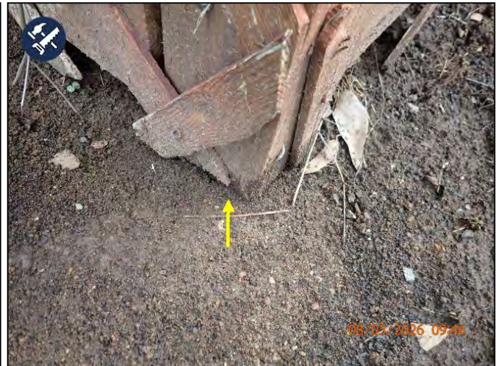
Wood-To-Ground Contact (Left Of Structure)
