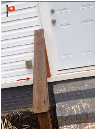
Missing Graspable Handrail(s)
