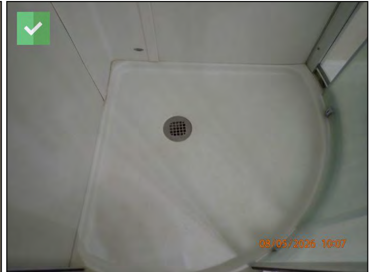
Main Drain Functioned
