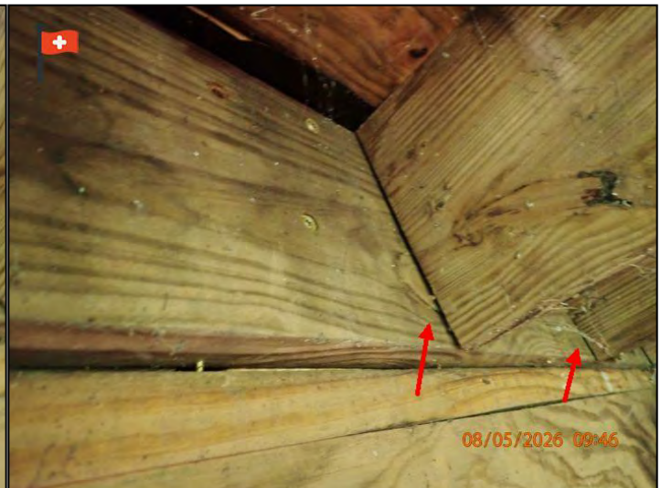
Missing Joist Hangers (Left Of Structure)
