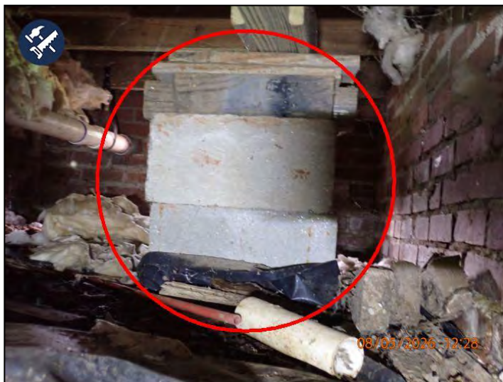
Dry-Stacked/Unprofessional Install (Multiple Locations)
