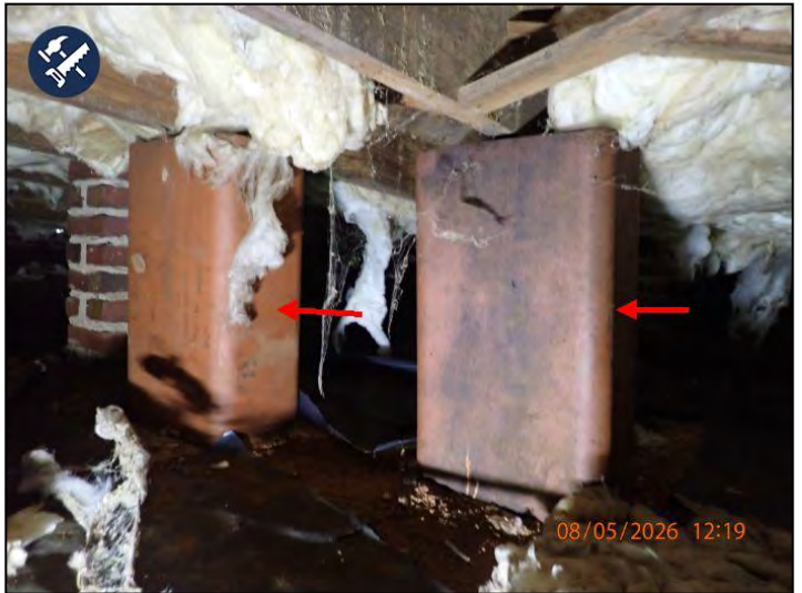
Unprofessional Install (Terracotta Pipes)
