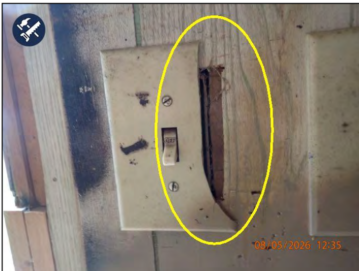
Damaged Cover(s) (Multiple Locations)
