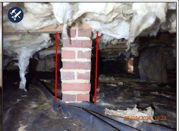
Leaning Pier(s) (Multiple Locations)
