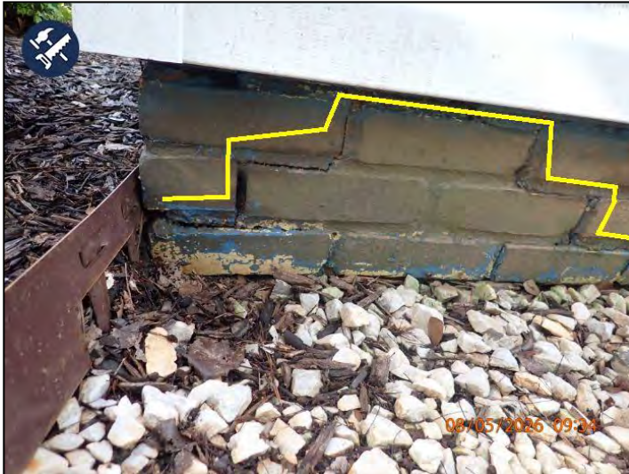
Step Crack(s) (Multiple Locations)
