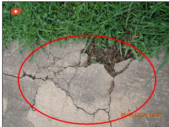
Walkway Has Cracking With Over 1/4" Differential (Tripping Hazard) (Multiple Locations)
