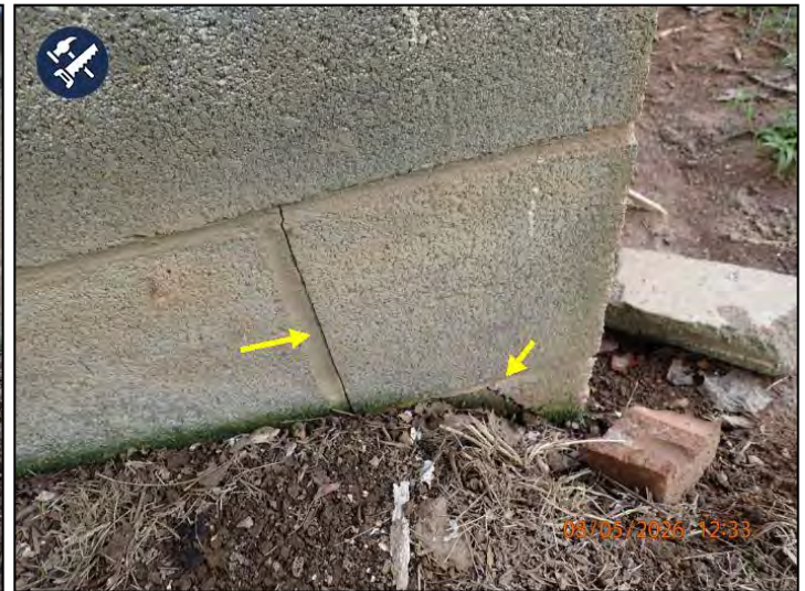
Step Crack(s) (Right Of Structure)
