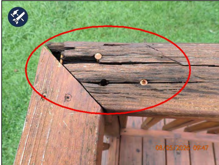
Significant Deterioration/Exposed Nails (Left Of Structure)
