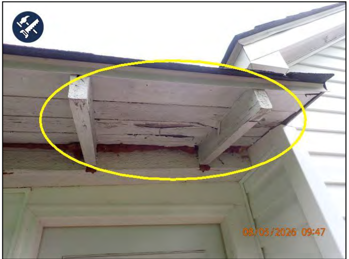
Damage/Deterioration (Multiple Locations)
