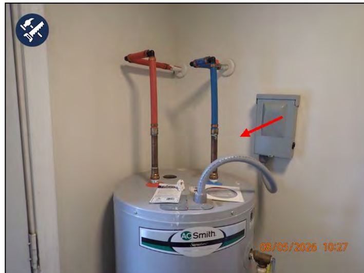
Expansion Tank Missing
