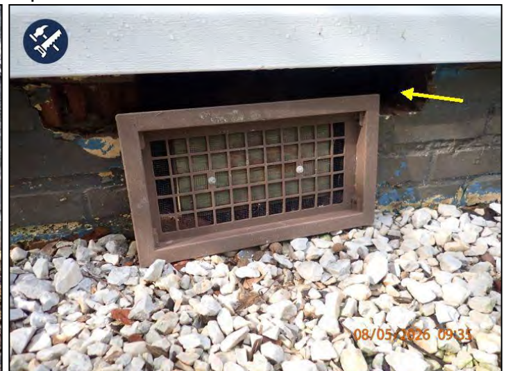
Unsealed Penetration(s) (Multiple Locations)
