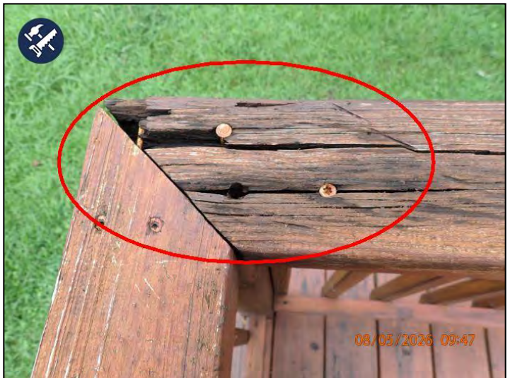
Significant Deterioration/Exposed Nails (Left Of Structure)
