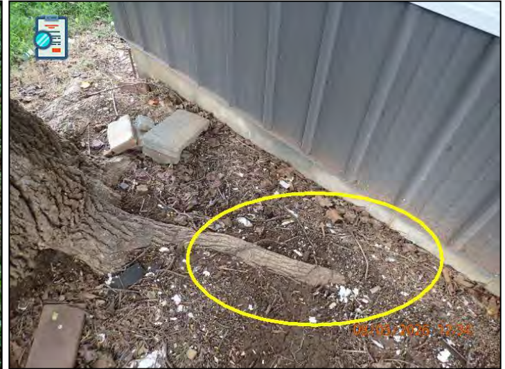
Tree Roots Close To Structure (Multiple Locations)
