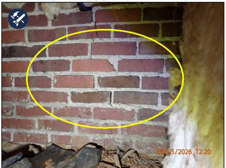
Settlement Crack(s) (Original Foundation Wall Between Kitchen/Dining Room)
