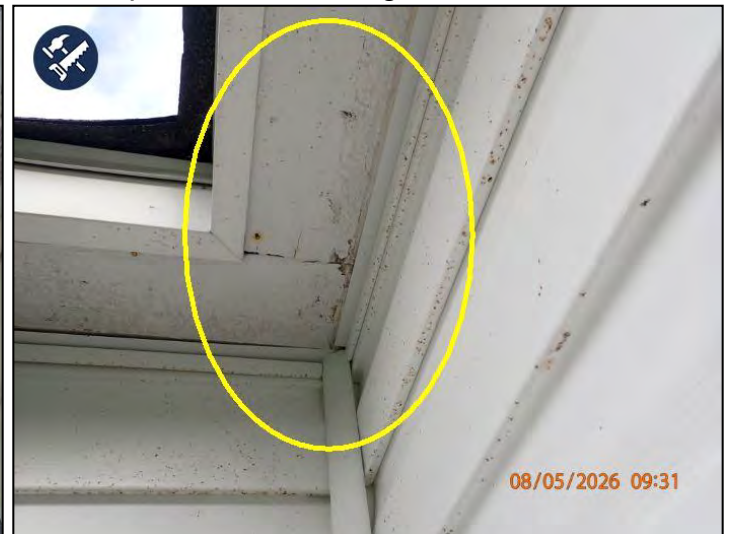
Damage/Deterioration (Multiple Locations)
