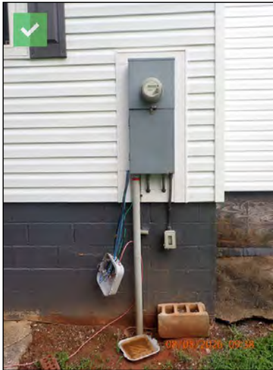
Underground Service Lateral: Rear Of Structure
