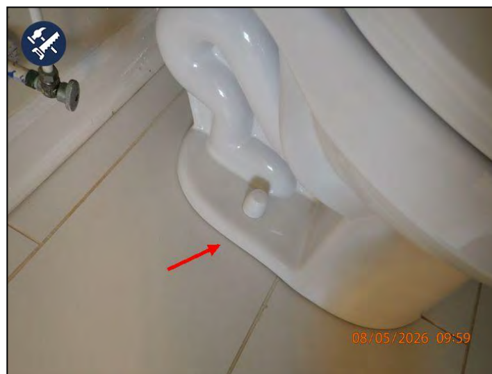
Loose (Primary Bathroom)
