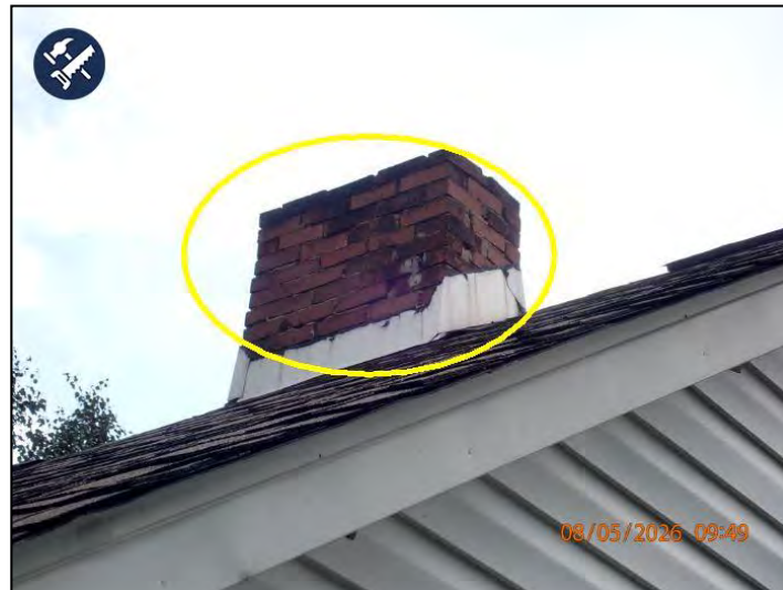
Significant Mortar Deterioration
