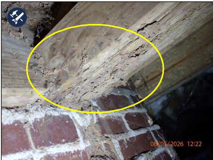
Evidence Of (WDI) Wood Destroying Insects/Organisms (Abandoned Chimney)
