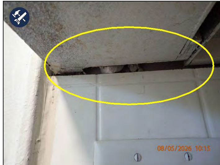
Unprofessional Install/Missing Trim (Multiple Locations)
