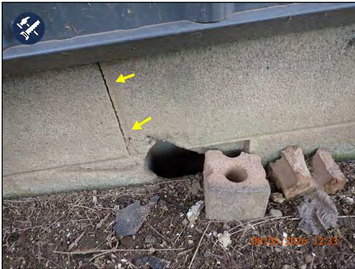
Vertical Crack(s) (Multiple Locations)
