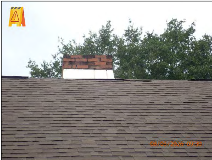
Abandoned Chimney (Could Not Determine If Properly Capped/Sealed)
