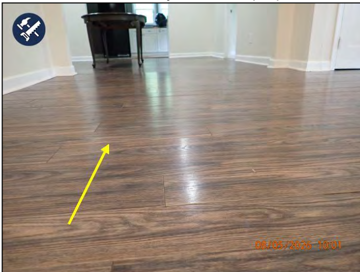
Not Level/Soft Sub Flooring (Multiple Locations)
