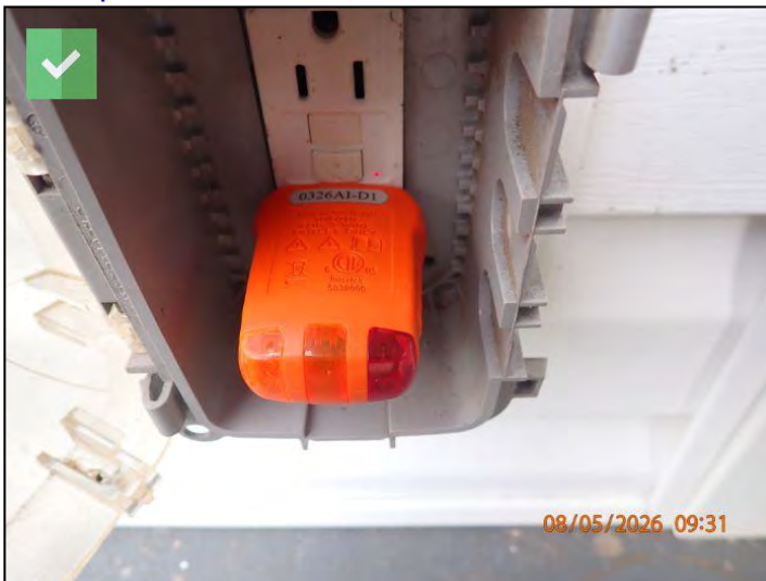
GFCI Reset Location For Exterior Receptacles: Within Each Receptacle
