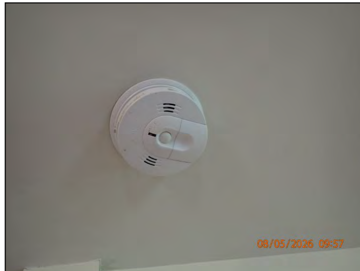
Combo Smoke/Carbon Monoxide Detector(s) Observed
