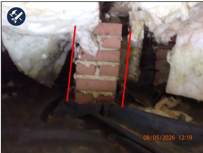
Leaning Pier(s) (Multiple Locations)
