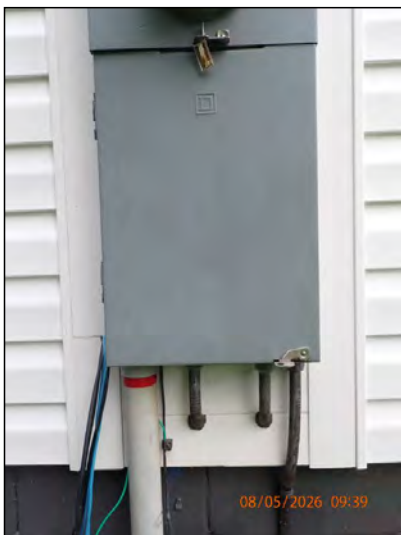
Main Electrical Panel Location: Rear Of Structure
