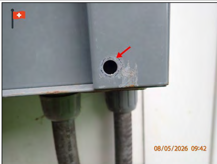
Missing Screw(s) (Main Panel)
