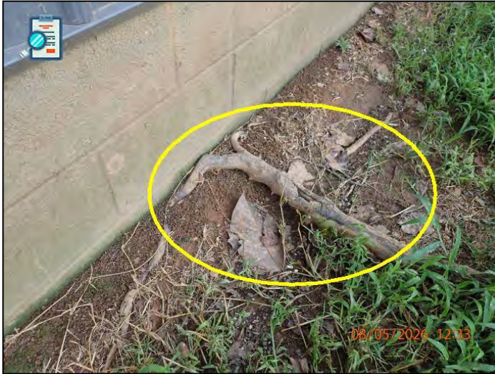
Tree Roots Close To Structure (Multiple Locations)
