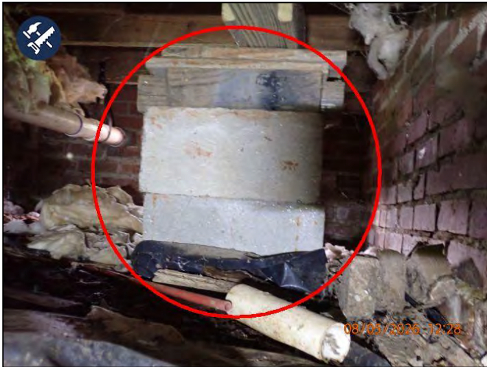
Dry-Stacked/Unprofessional Install (Multiple Locations)
