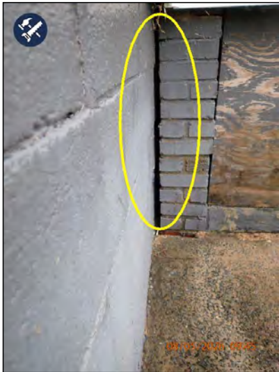
Unsealed Penetration(s) (Multiple Locations)
