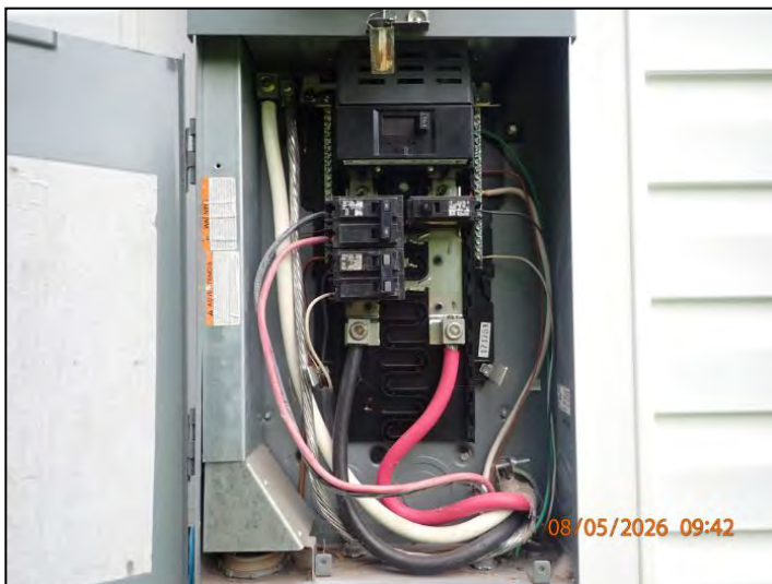
Main Electrical Panel Location: Rear Of Structure
