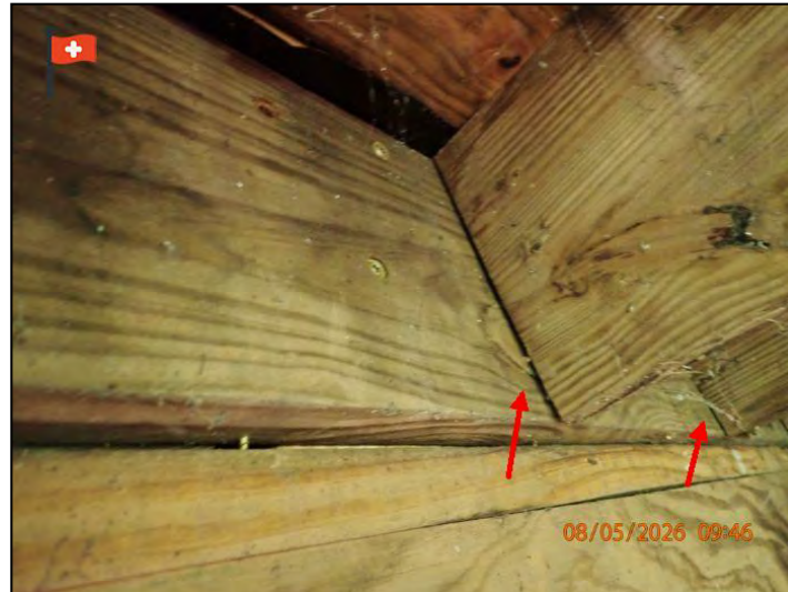
Missing Joist Hangers (Left Of Structure)
