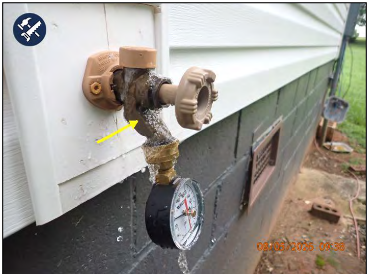
Leak At Valve
