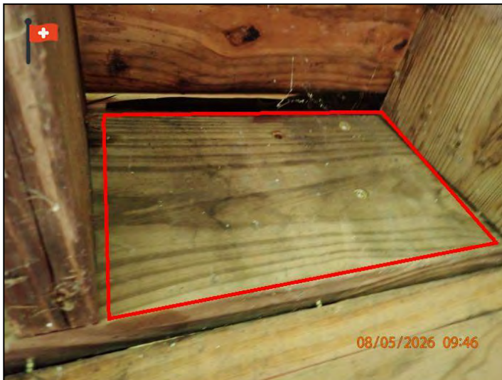
Inadequate Hardware Used In Ledger Board (Left Of Structure)
