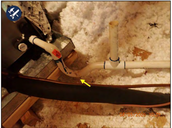
Trap Missing Insulation
