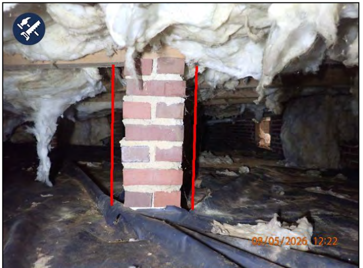
Leaning Pier(s) (Multiple Locations)
