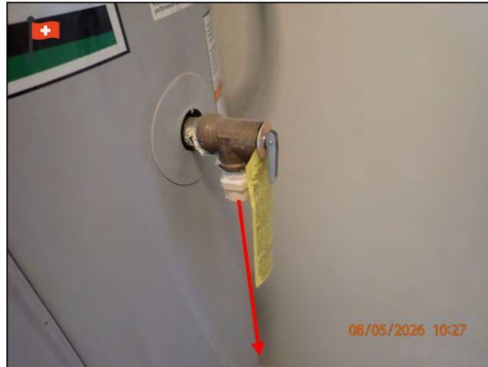
Missing Discharge Pipe
