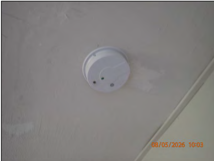
Smoke Detector(s) Present
