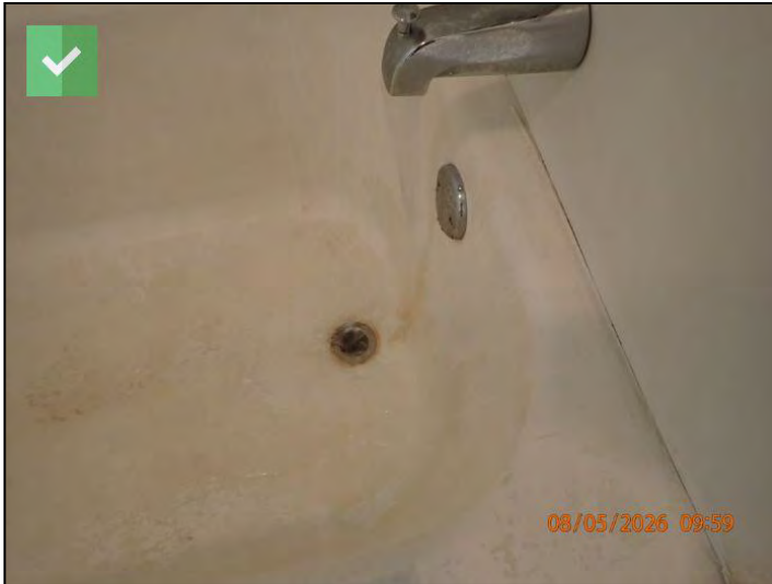
Main Drain Functioned
