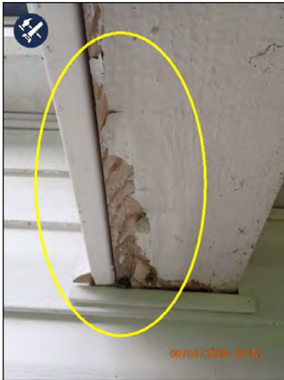
Damage/Deterioration (Multiple Locations)
