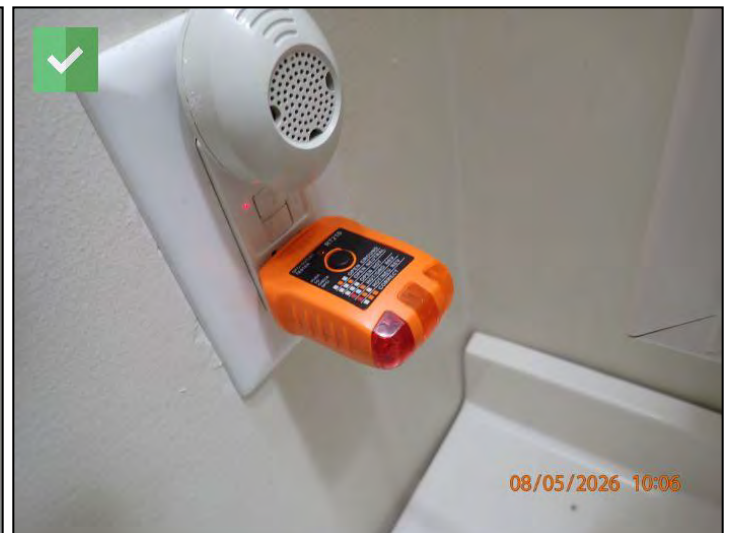
GFCI Reset Location For ALL Bathrooms: Guest Bathroom
