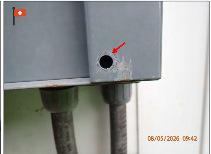
Missing Screw(s) (Main Panel)
