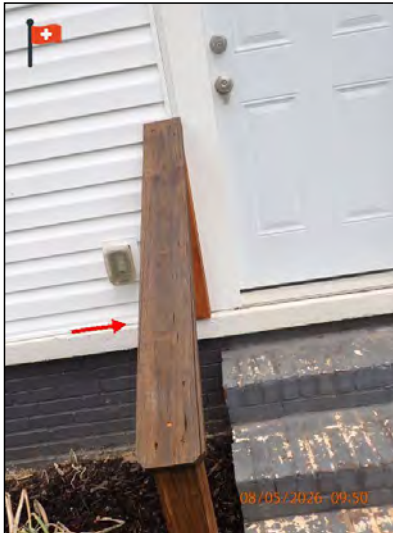
Missing Graspable Handrail(s)
