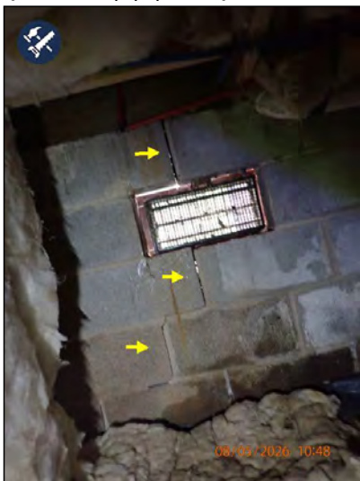
Settlement Crack(s) (Right Of Structure)
