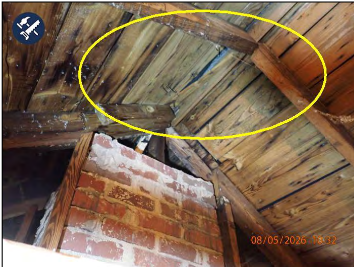
Damaged Sheathing (Multiple Locations)
