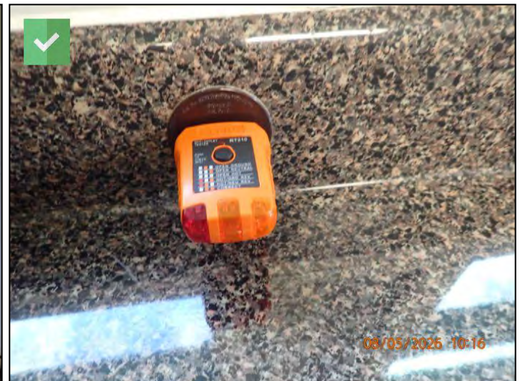
GFCI Reset Location: Electrical Panel
