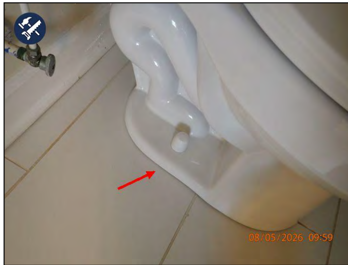
Loose (Primary Bathroom)
