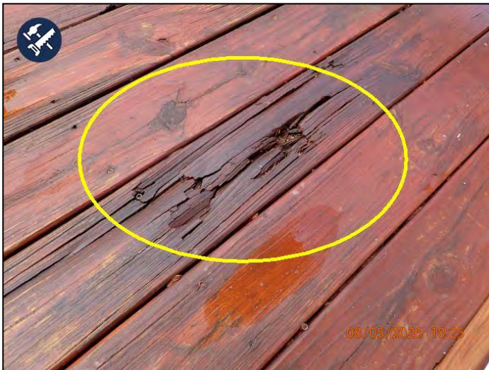
Deterioration (Multiple Locations)
