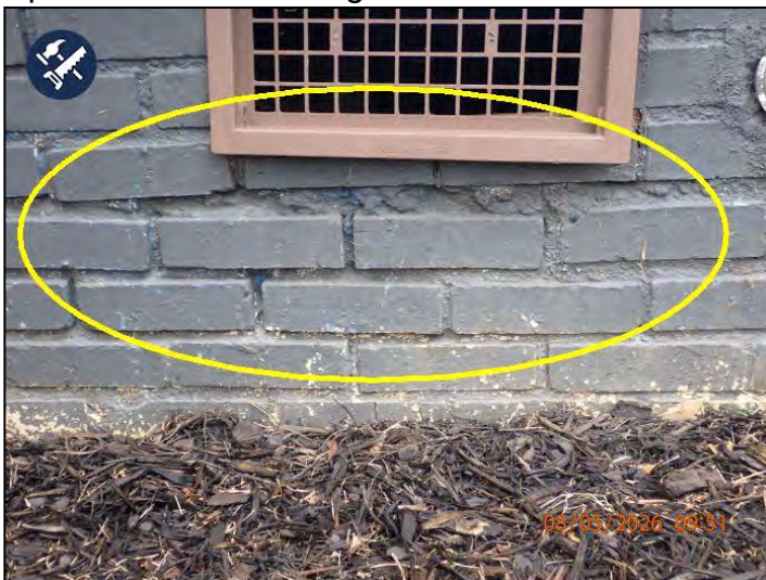
Past Repairs (Unable To Determine If Professional)
