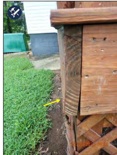
Deterioration/Warping (Multiple Locations) (Left Of Structure)
