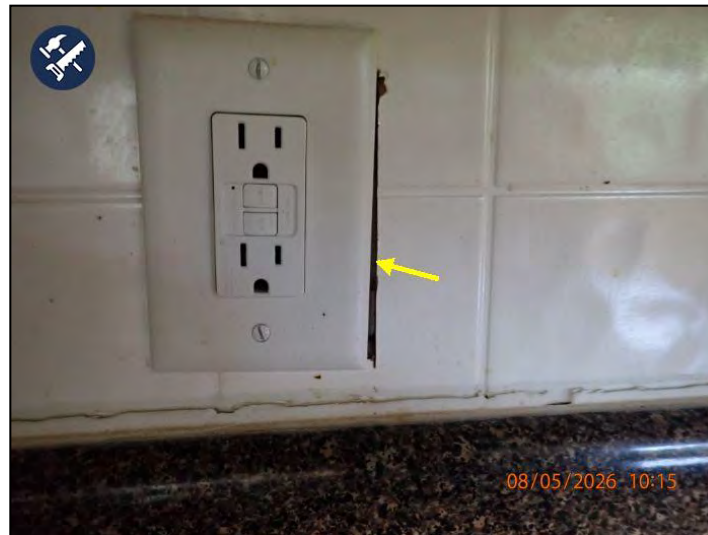
Loose/Improperly Installed Outlet(s)
