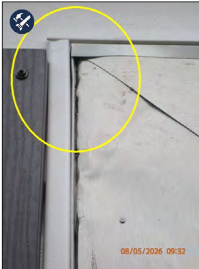
Damaged Trim (Multiple Locations)
