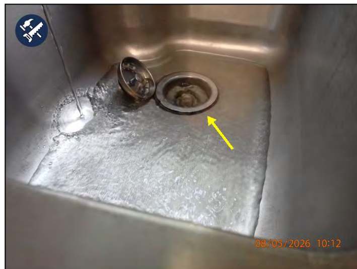
Slow Drain/Clogged (Both Sinks)
