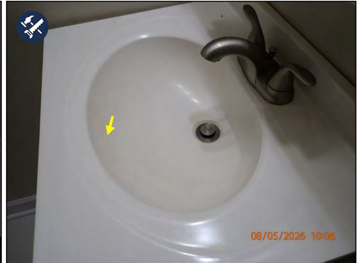
Missing Overflow Drain (Guest Bathroom)
