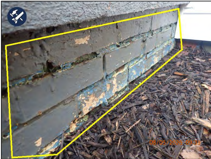
Deterioration (Multiple Locations)
