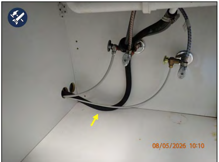
Missing High Loop
