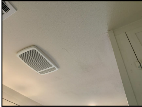
Bath fan was functional
