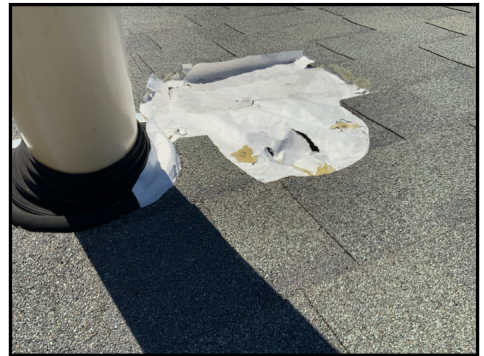
Hole in roof
