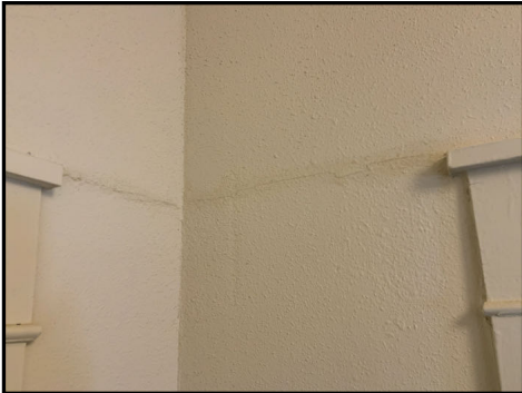
Cracks in hallway
