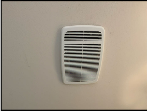
Bath fan was functional
