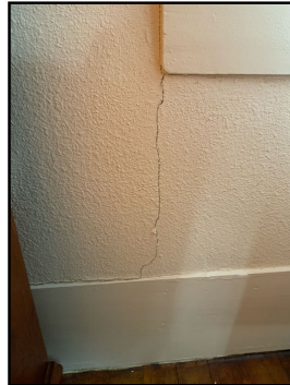
Crack in front bedroom
