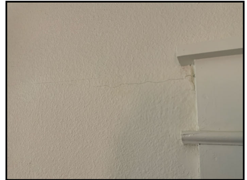
Crack by front door
