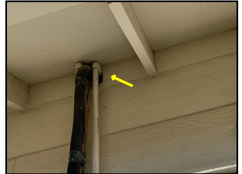
Hole needs sealed up
