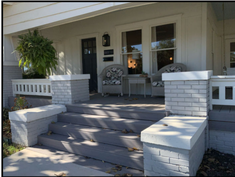
Handrail is missing
