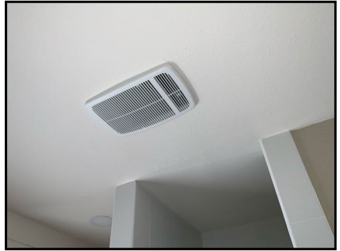
Bath fan was functional
