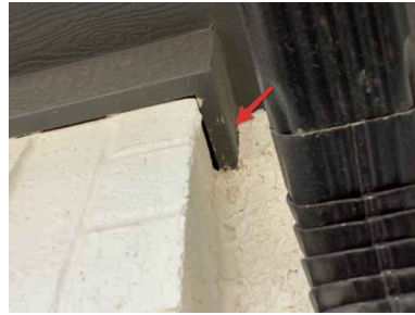
Front right corner trim gap
