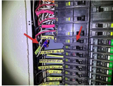
Large garage sub panel
