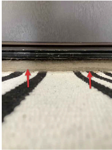
Bottom of front door threshold
