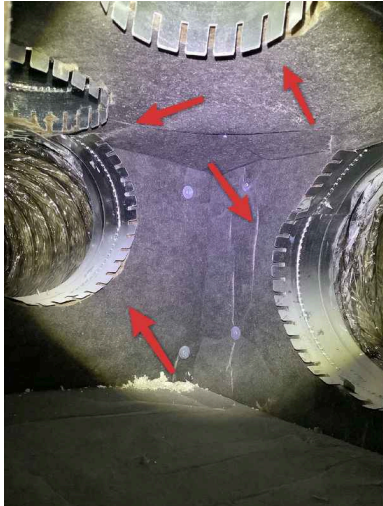
Flanges not implemented
