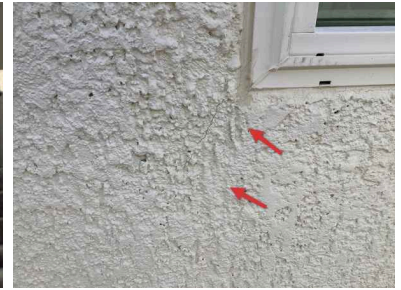
Right side dining room. Cracking
