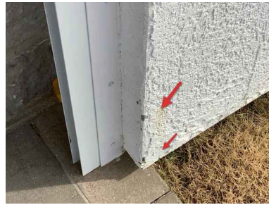
Minor damage at back patio on lower walls
