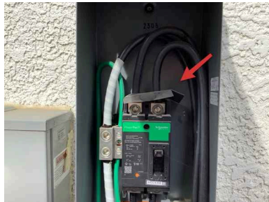
Not installed properly
