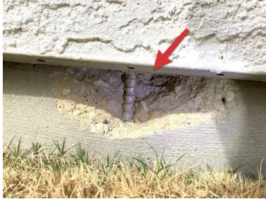
Lower plate bolt exposed on left rear
