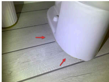
Front suite toilet leaking at base
