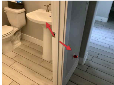
Outside powder room. Within 6ft of sink
