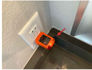
Front suite. Not resetting properly every time
