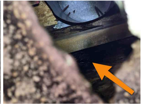
Wet Sheathing - Long term water damage
