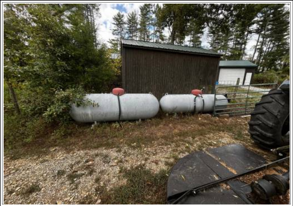
LP Gas Tanks
