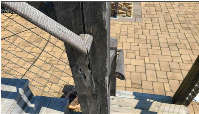
2.4 Item 3(Picture) exposed screw at edge presents sharps hazard
