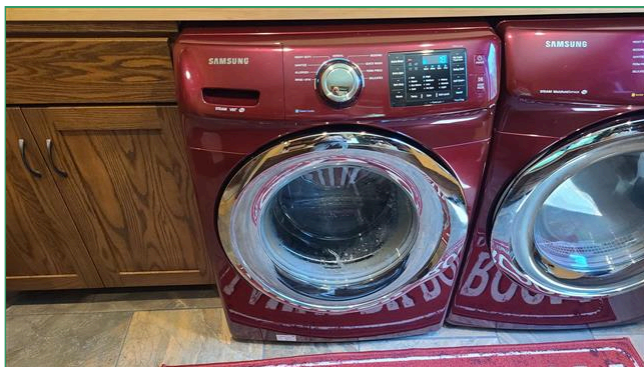
4.14 Item 1(Picture) unable to view supply lines and drain due to countertop configuration
