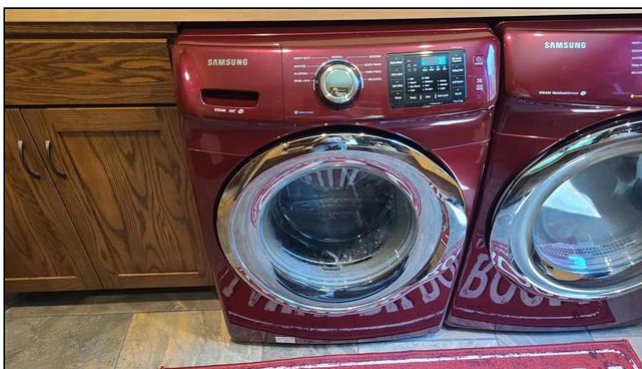
4.14 Item 1(Picture) unable to view supply lines and drain due to countertop configuration
