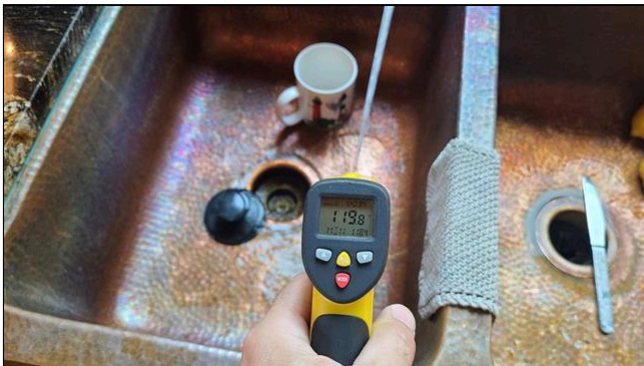
8.2 Item 1(Picture) Temperature at kitchen sink
