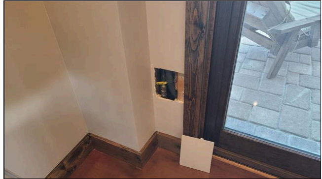
2.6 Item 4(Picture) access point for rear left corner located inside panel of rear left corner basement bedroom
