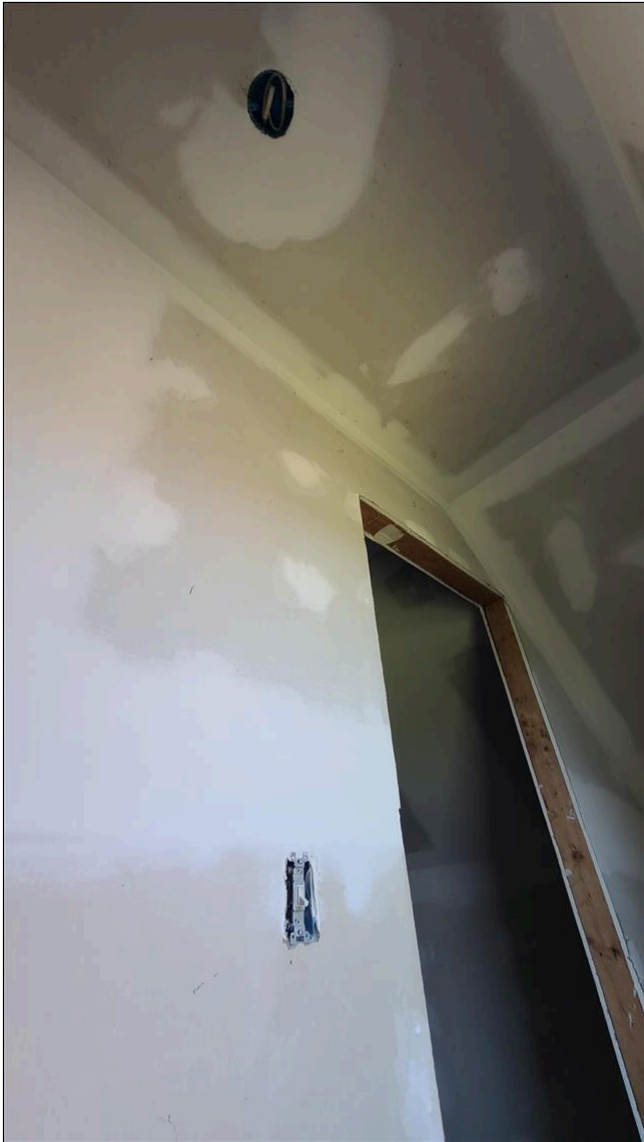
3.2 Item 1(Picture) upper level of garage stairwell - light switch and open junction box for light fixture
