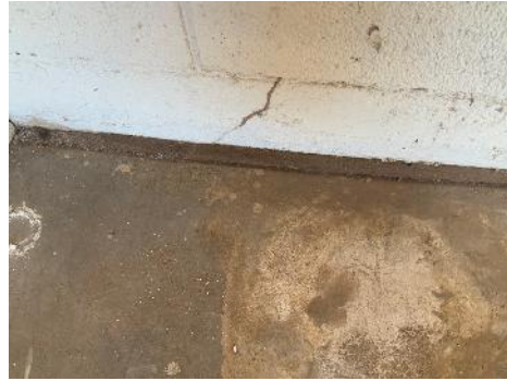
Subterranean termite tube exterior foundation
