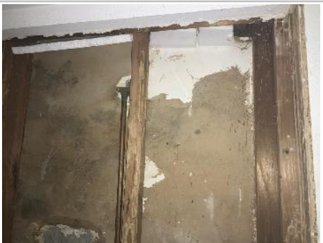
Subterranean termite evidence entry hall
