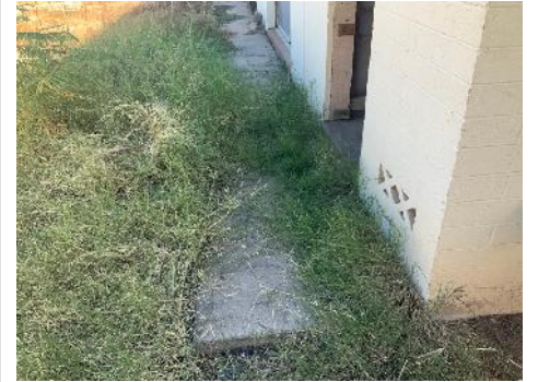
Plants abutting structure
