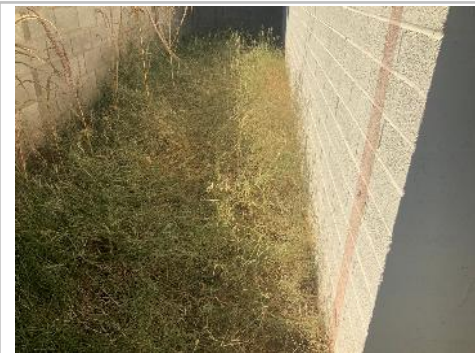
Plants abutting structure
