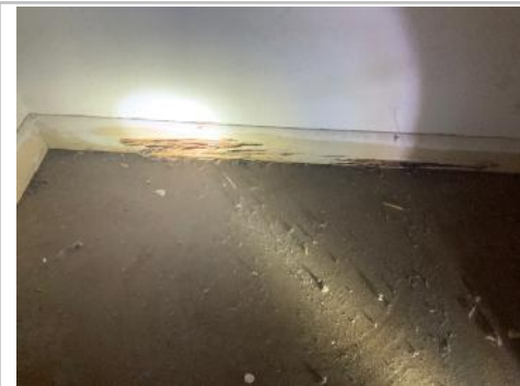
Subterranean termite damage southern bedroom
