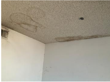
Water stains bedroom ceiling
