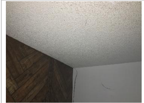
Subterranean termite tubes family room
