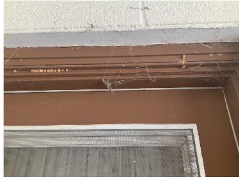
Subterranean termite tubes carport door frame
