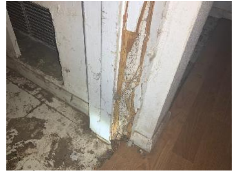
Subterranean termite damage pantry
